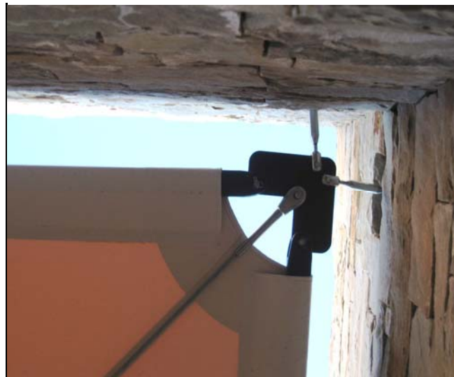
FIGURE 4 Burnside Wall Anchorage
